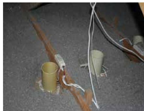
Incorrect usage of combustible PVC Pipes as restraint. This is a potential fire hazard.
