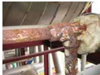
Corrosion under insulation
